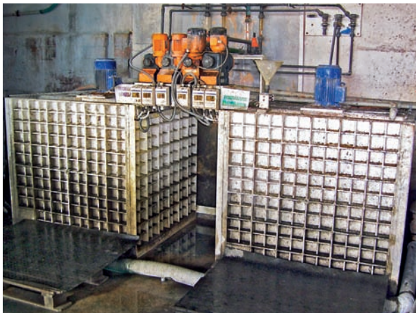
Photo 1. Coagulant/flocculant dosing station
