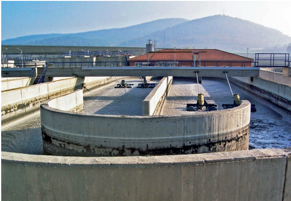
Photo 12. Oxidation ditch in operation
