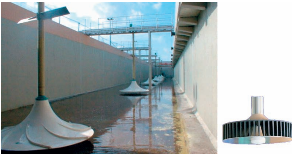
Photo 11. Submersed turbine aerators in oxidation ditch
