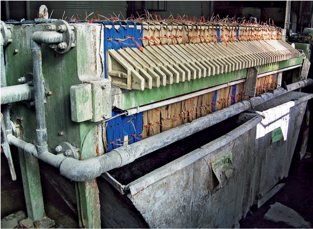
Photo 5. Recessed-plate filter press with container for dewatered sludge
